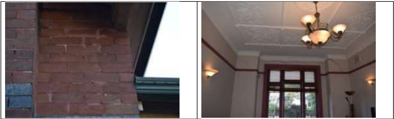
Figure 3: Detailed view of the front façade showing repair works previously conducted (left) and an interior view of a front room within the residence, with a large horizontal crack visible directly underneath the cornice detailing (right).
