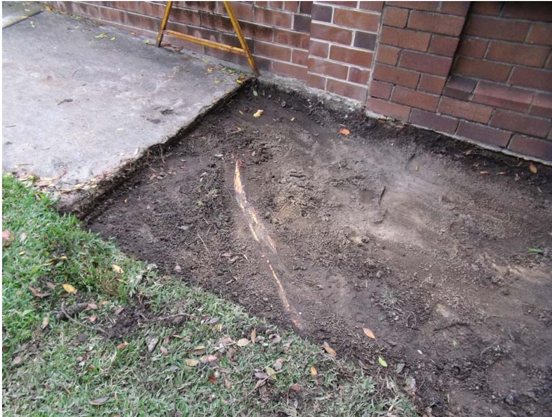
Very large fig tree root travelling into the front yard area of 13 Helena Street
