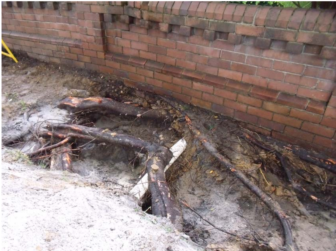
Mass of large matted fig tree roots damaging footpath, stormwater pipe and brick fence
