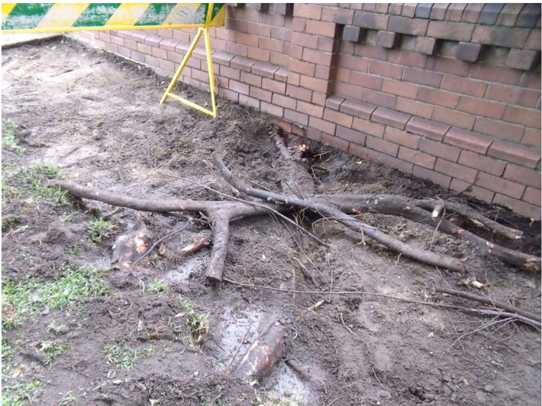
Large numbers of fig roots extend across the entire adjacent property frontage
