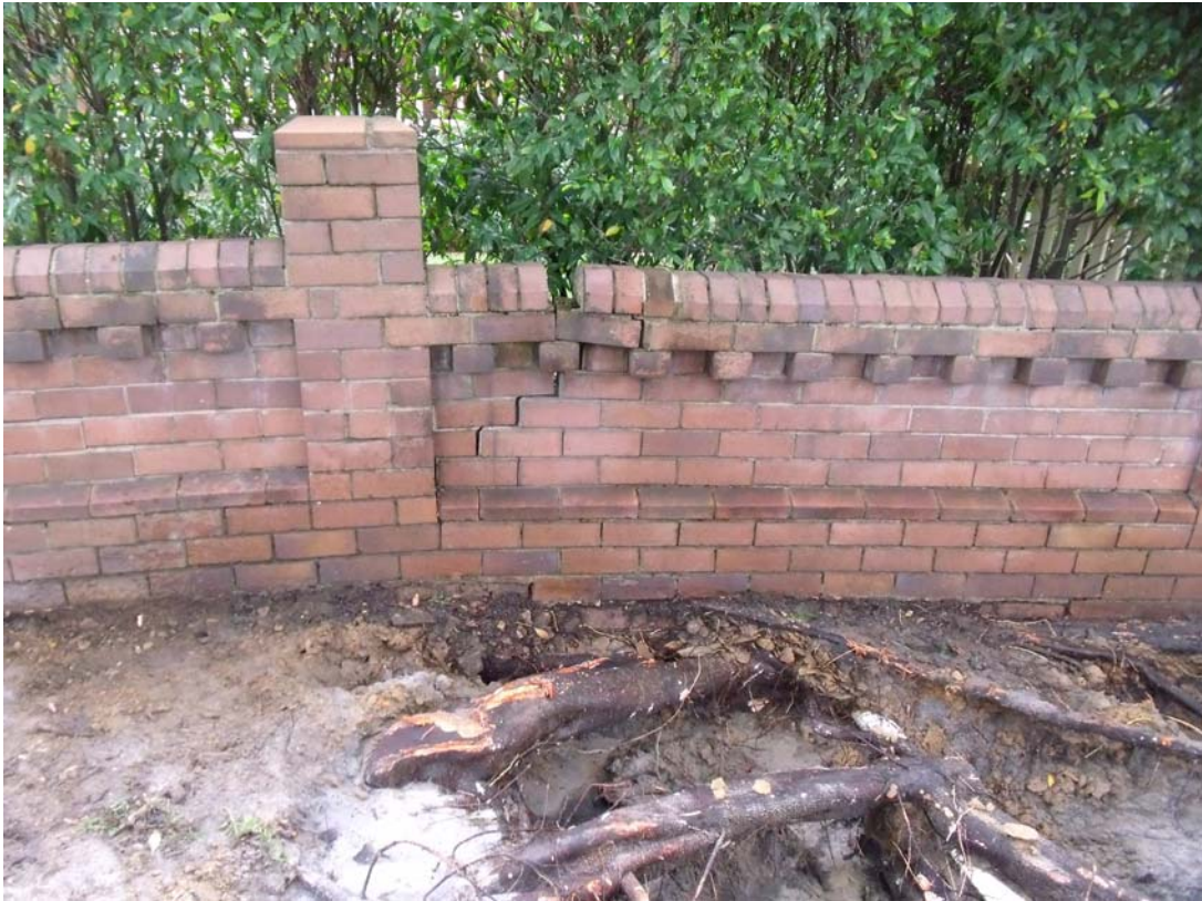
Front brick fence at 11 Helena Street has been severely damaged by fig tree roots
