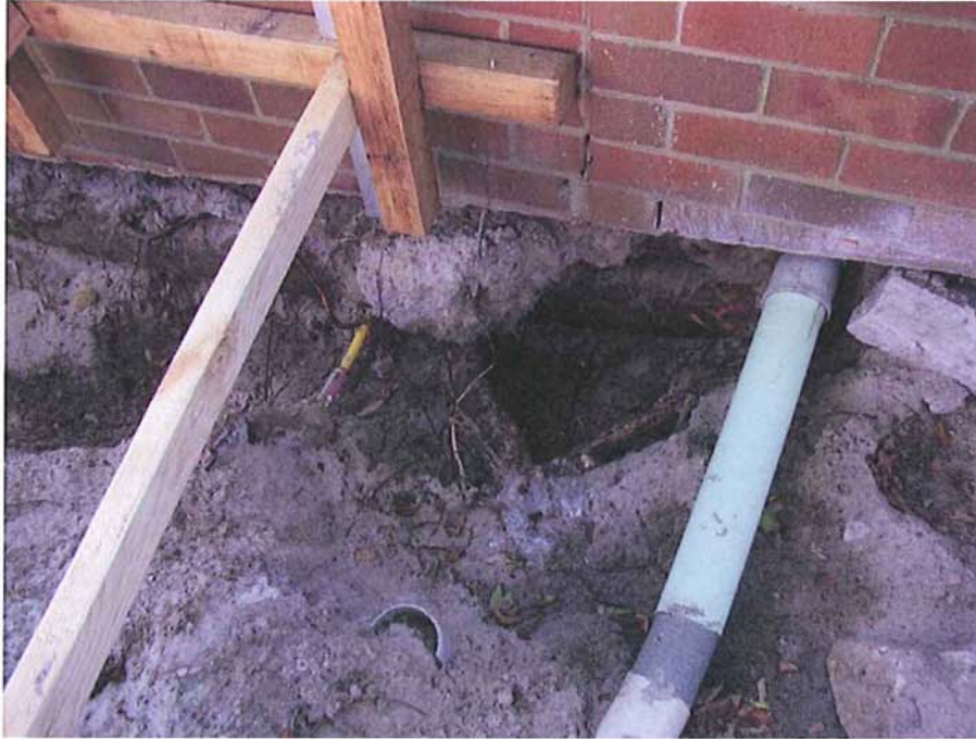
Roots growing around gas pipe and stormwater pipes adjacent to front of property
