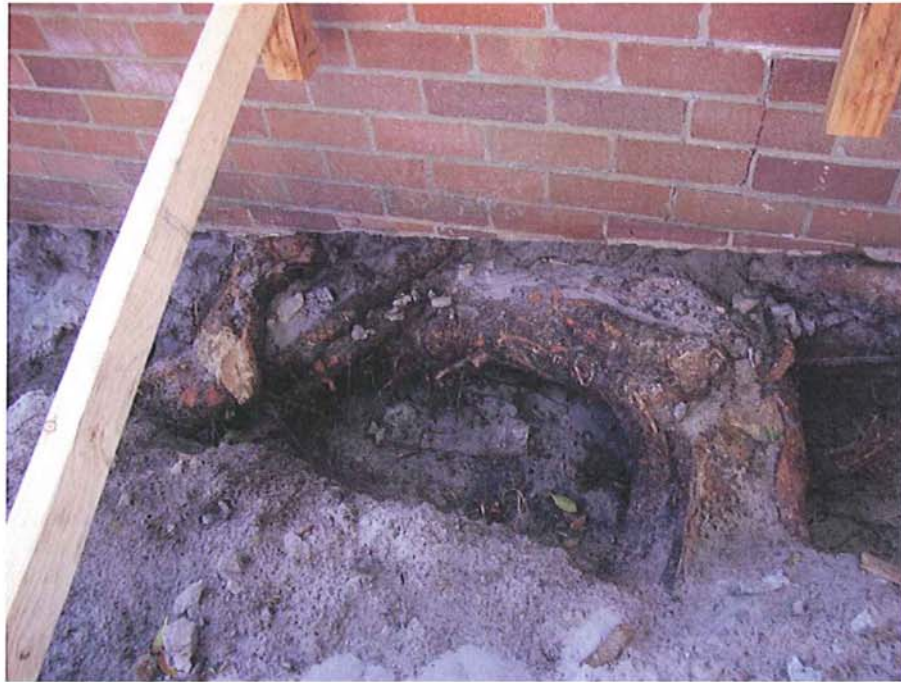
Large tree root (200mm diam) growing under brick wall and into property
