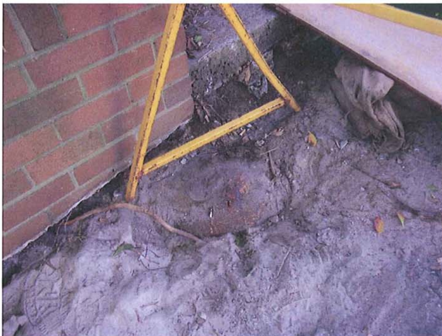
Large tree root growing under brick fence and deviating into property
