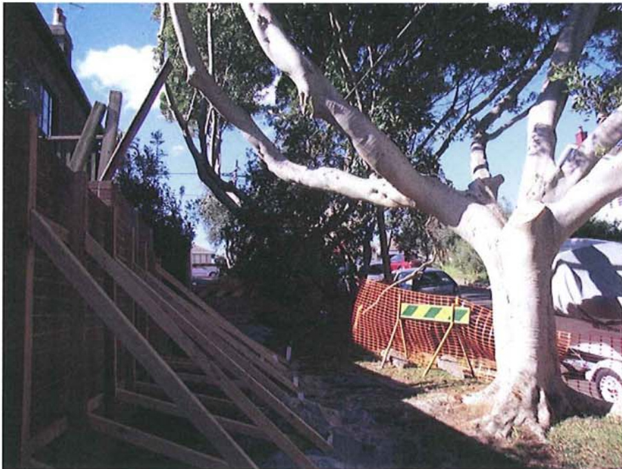
Impact of trees on adjacent infrastructure along eastern end of Athol Street
