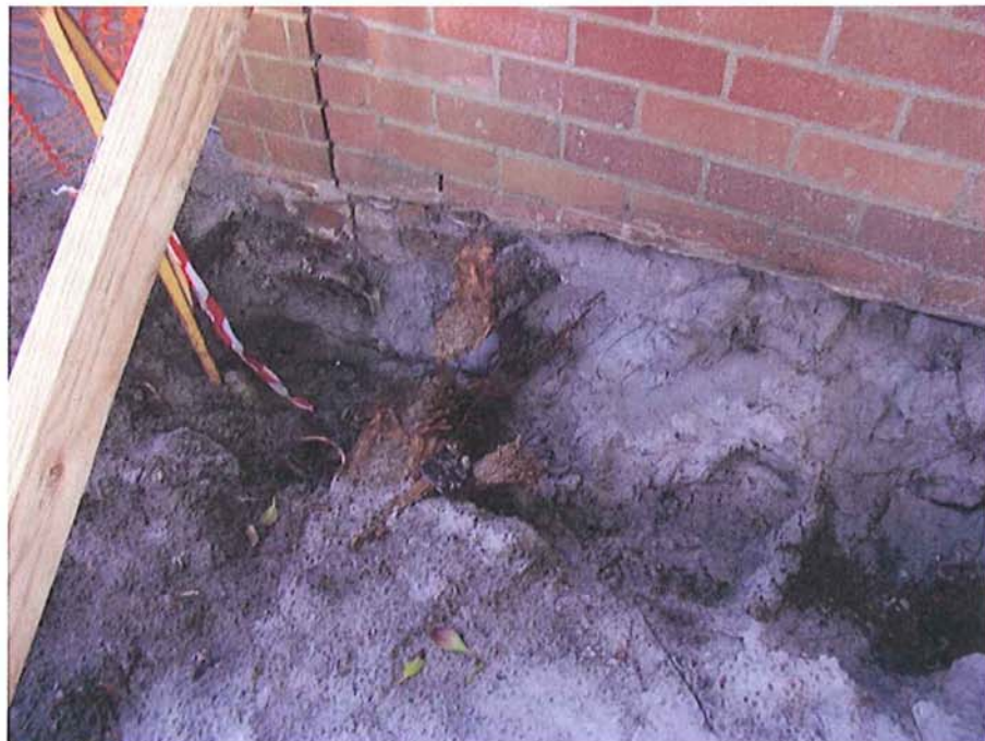
Tree root growing under brick wall and causing cracking
