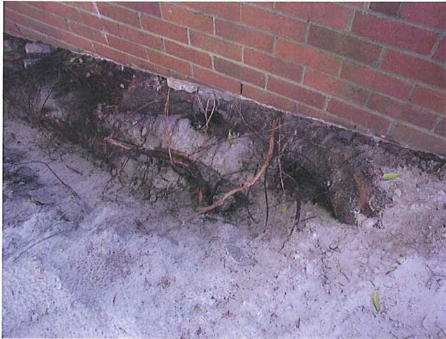
Roots running underneath brick fence and undermining adjacent footpath
