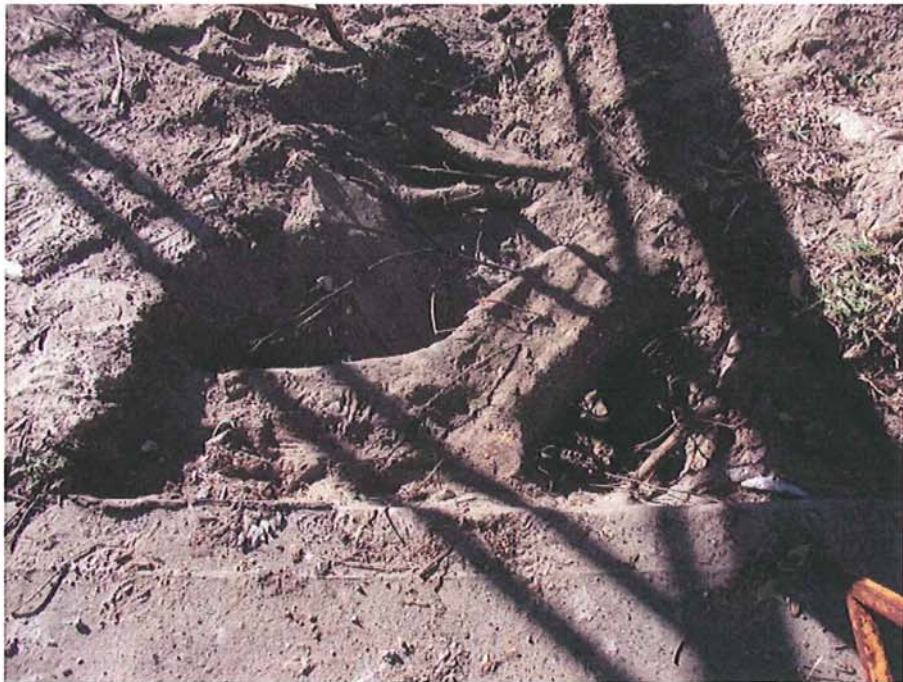
Large tree root growing under driveway into property
