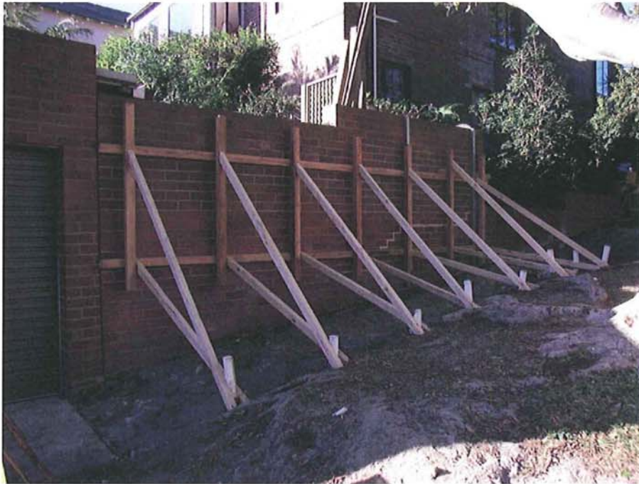
Damaged brick wall has had to be braced because of tree root damage
