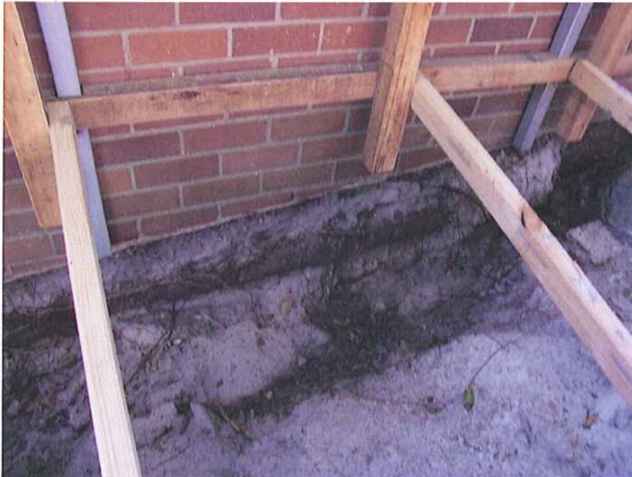
Tree roots snaking underneath eastern section of brick wall
