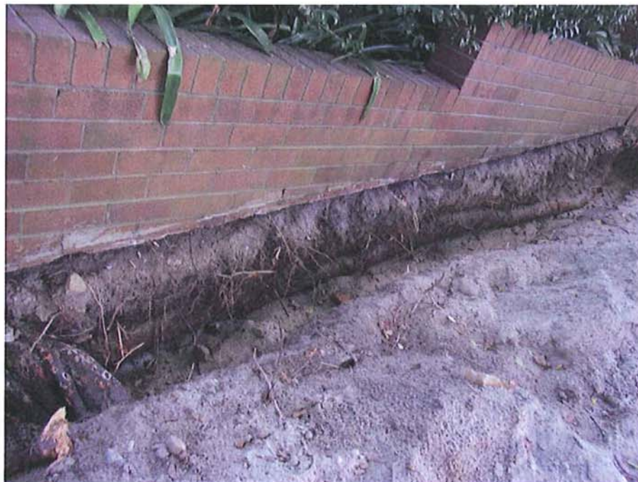
Tree roots snaking along section of brick fence and entering property
